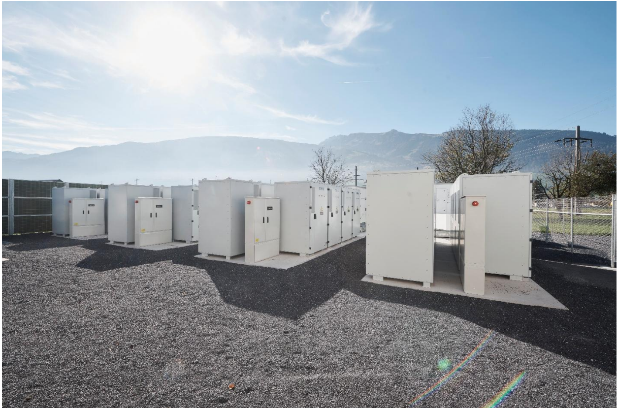
Batteriespeichersystem in Mels/SG
